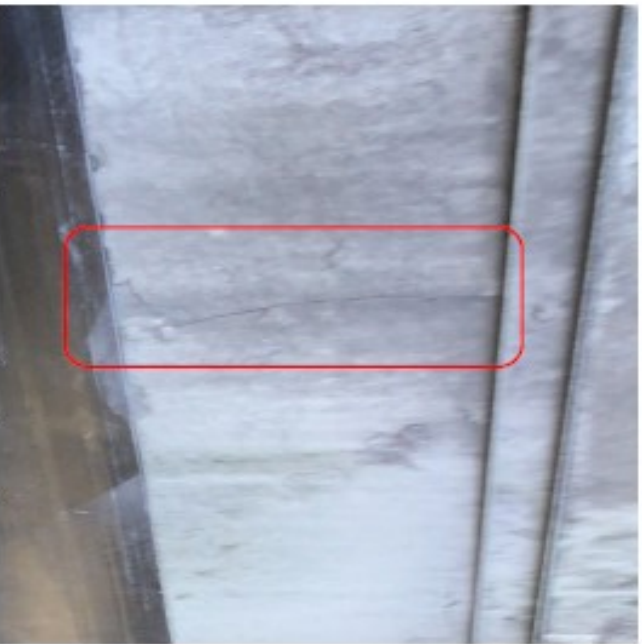
Crack on a cement board panel.
