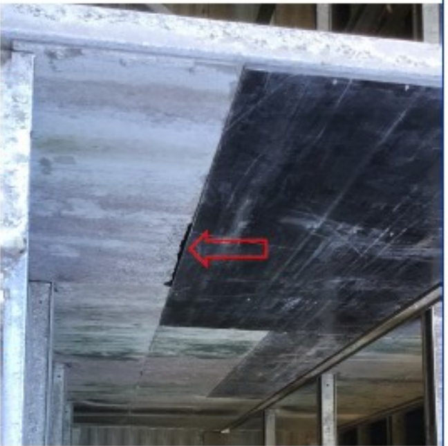
Degradation on the top edge of a cement board wall panel.
