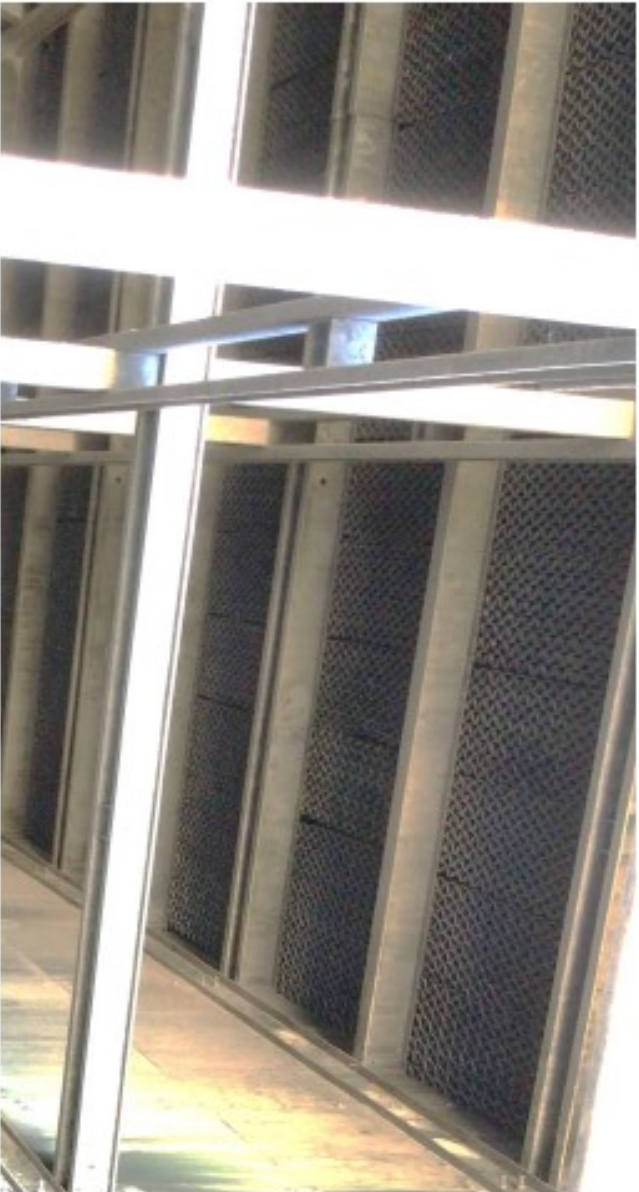
Underside of fill packs. Some gaps have formed between the brittle bottom layer fill packs.
