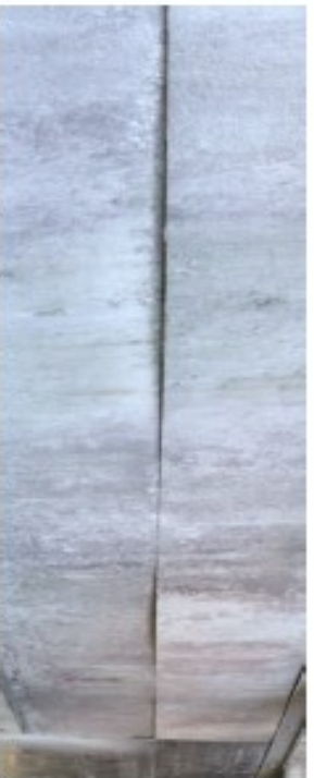
Example of cement board warping at the seams between the supporting structure.
