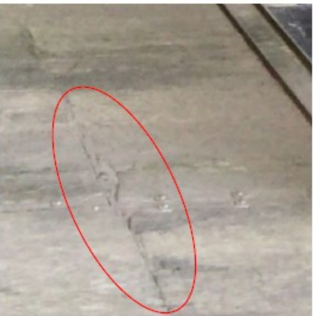
Degradation on the edges of the cement board panels.
