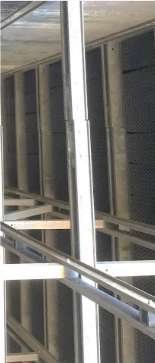
Underside of fill packs. Some gaps have formed between the brittle bottom layer fill packs.
